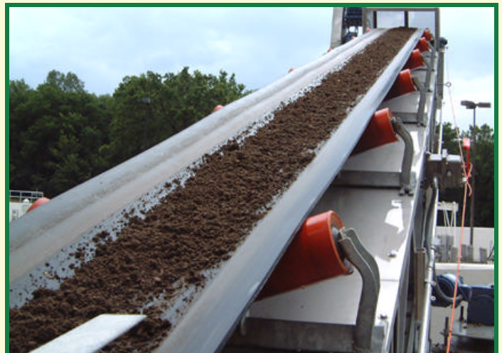
Lime Stabilization takes less than five-minutes to produce guaranteed Class B Stabilization
