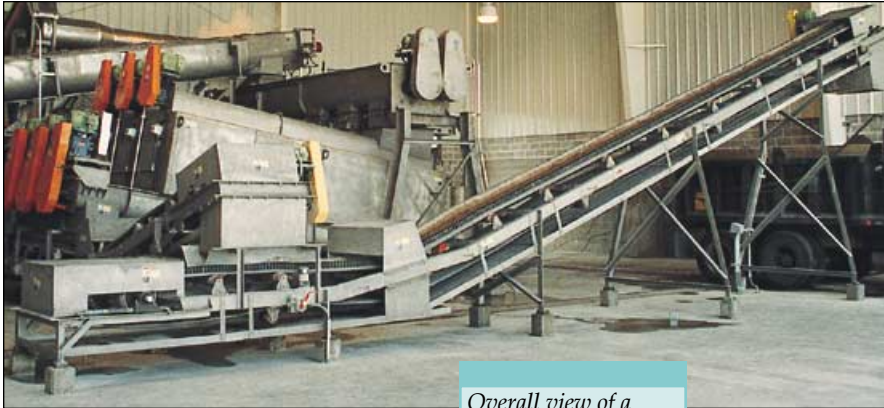
Overall view of a 1.5 dry ton per hour system utilizing a ThermoFeeder™, ThermoBlender™ and Pasteurization Vessel.
