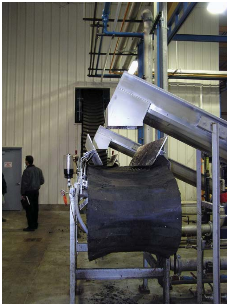
Left: Dewatered cake is discharged onto a Serpentix Conveyor that elevates the dewatered cake to the ThermoBlender in an adjacent room.
