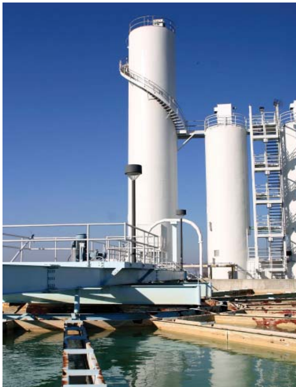
Left: Existing softening basin is one of four dosing points for the lime slurry.
