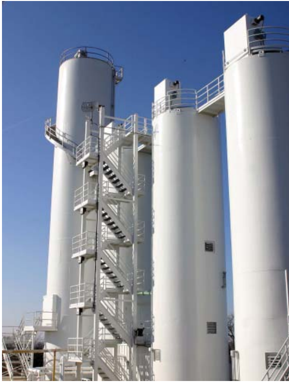
Left: Three 12 foot diameter storage silos with original access stairway. RDP furnished a new spiral stairway, in the background, from the top of the existing stairway to the top of the new 14 foot diameter silo.
