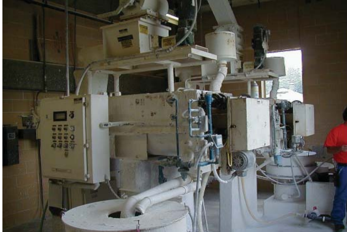
Left: One of two existing continuous paste type slakers replaced with a Tekkem Slaker.
