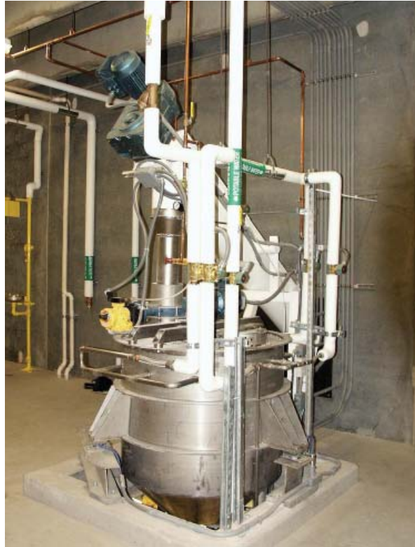
Above: Water and air piping shown for proper operation of the Tekkem Slaker.
