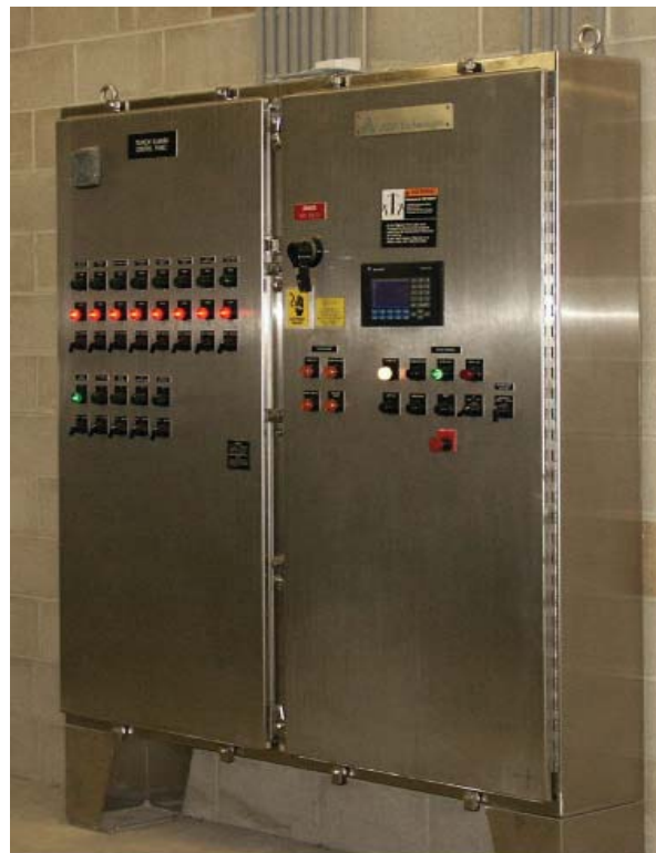
Above: The Tekkem System Control Panel is a NEMA 4X stainless steel, double door enclosure with an Allen-Bradley PLC with a Panel View Screen.
