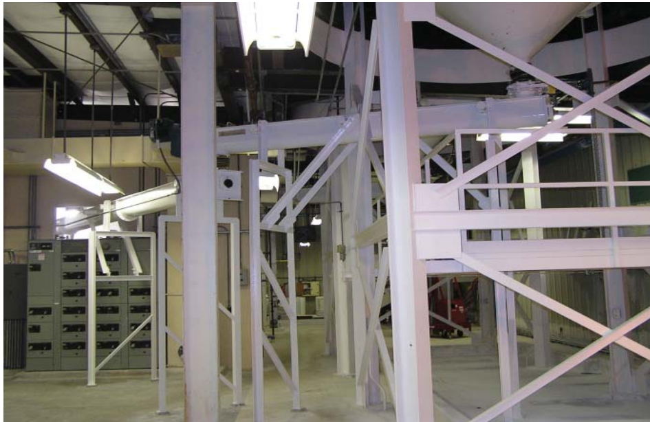
Above: The Tekkem System included two new lime transfer screw conveyors to convey the lime to an adjacent building room with the Tekkem Slakers.
