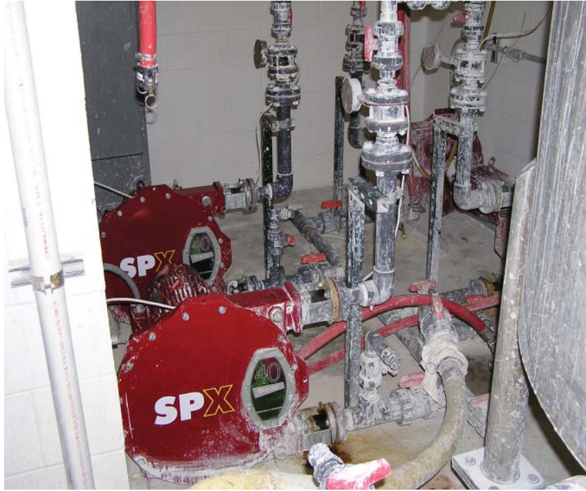
Left: Hose pumps deliver lime slurry from the Slurry Aging tank portion of the Tekkem Slaking System. See lime slurry discharge point below at each softening clarifier.
