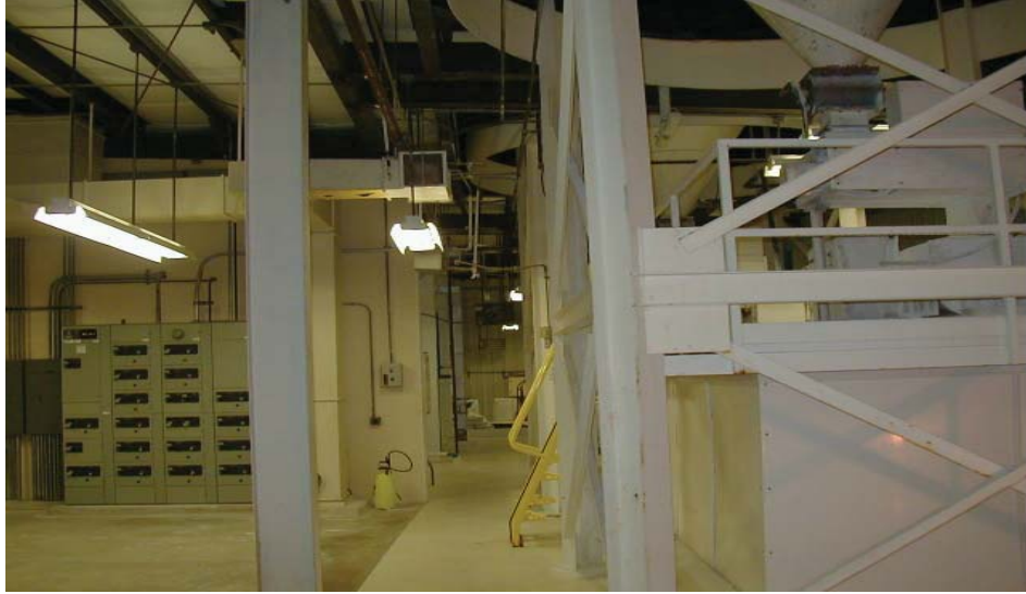
Above: Original continuous paste slaker located beneath the quicklime bulk storage silo with gravity lime slurry feed to the clarifiers.
