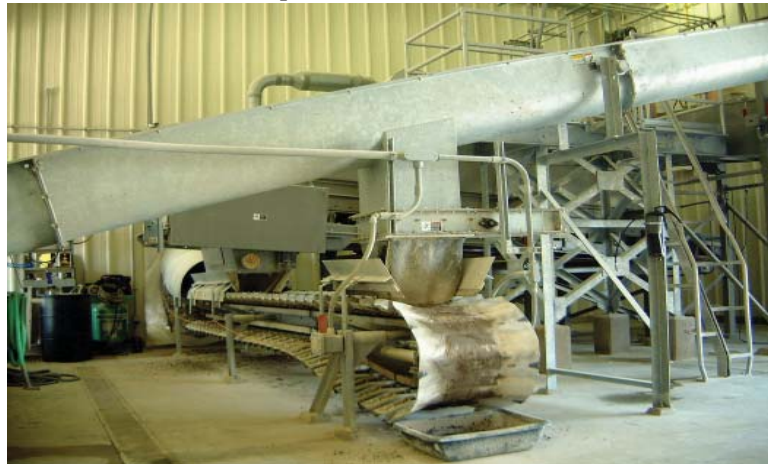
Above: The screw conveyor intermediate discharge point provides a simple method of bypassing the Pasteurization System.
