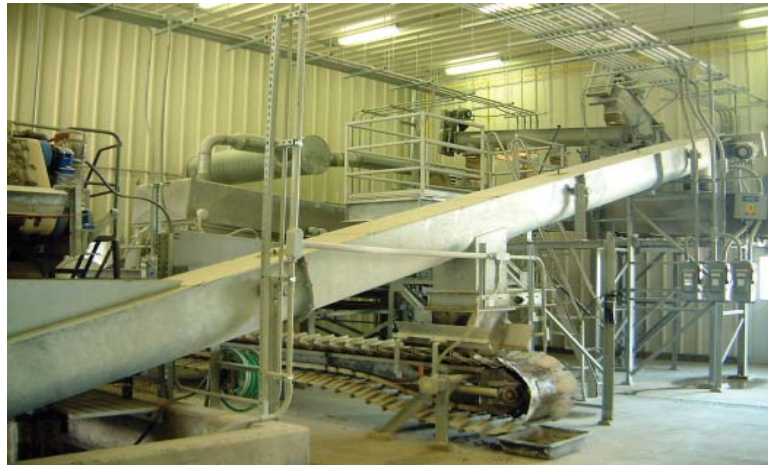
Above: The inclined sludge cake screw conveyor moves the 19-20% BFP cake to the inlet point on the ThermoBlender.
